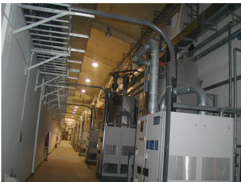
The plant realized at Shangai covers the bottle production in PET for one of most largest areas in China.
