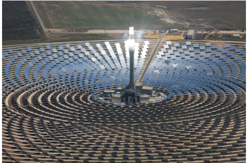
2650 mirrors focus and send the sun's heat to the 140 meter high tower's receptors in an area the size of 260 football pitches. This innovative energy production plant using renewable sources is capable of producing 400MWh a day.
